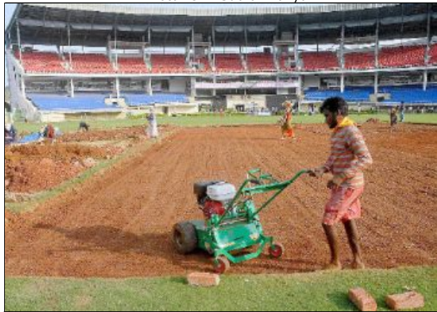
For a strong wicket: Work in progress at the cricket pitch at the ACA-VDCA Stadium in the city.
