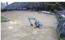
Completion of the drainage and laying of the growing medium on top
